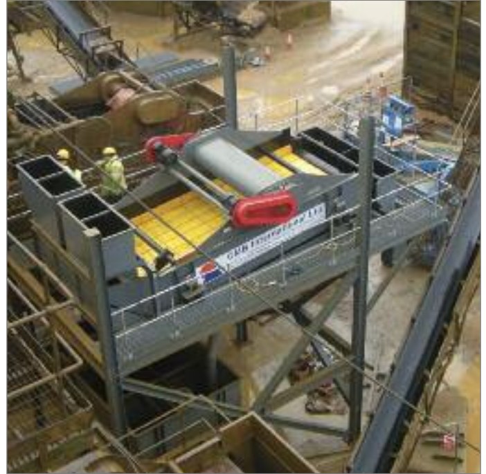
CMB de-watering screen installed at Lafarge, Hertfordshire. This screen was designed to work within a MEP sand plant.
