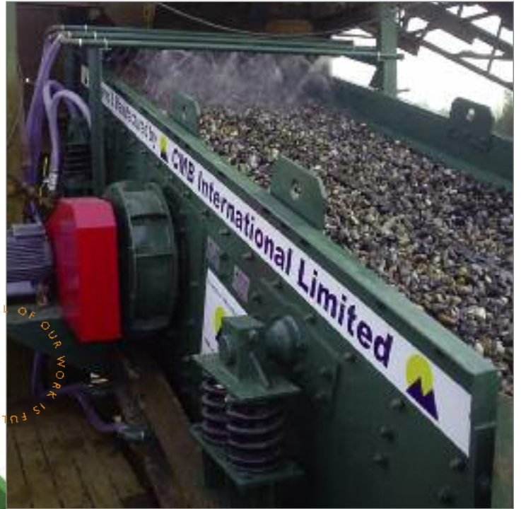
1.8m x 5m double deck screen working in a sand and gravel plant, Dereham, Norfolk.
